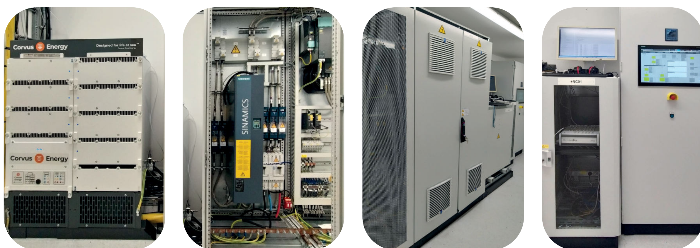
Figure 2: Battery system, power electronics units (two middle photos), EMS and the control cabinet incorporating the Human Machine Interface (HMI) of the MAN ES battery container (from left to right).
